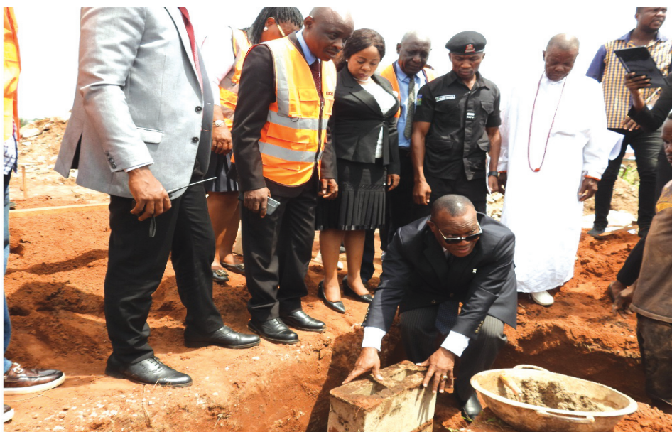
GROUND-BREAKING: Edo State Chief Judge, Hon. Justice Joe Acha laying the foundation at the ground-breaking ceremony for the Abudu High Court Complex, Edo State, last Tuesday. Looking on is Chairman, Edo State Oil and Gas Producing Areas Development Commission, EDSOGPADEC, Pastor Kennedy Osifo and others.
