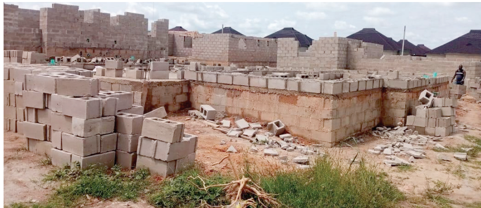
• Another destroyed project
