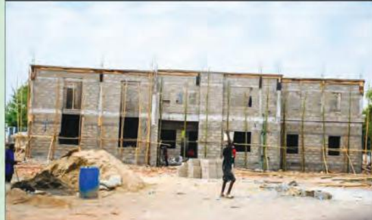
Ongoing construction of the office of the Secretary to the State Government
